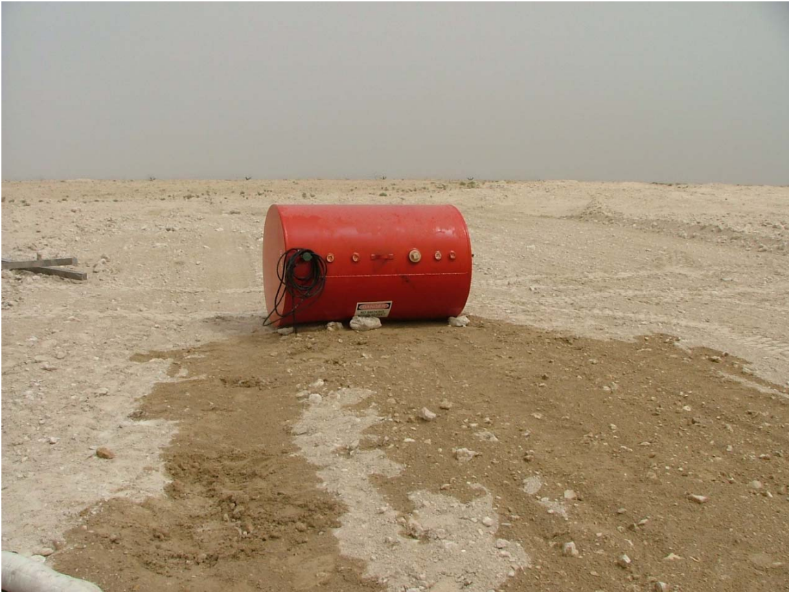
Figure 1 Diesel Fuel Tank Leak and Spill
